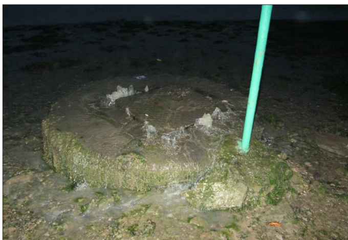
Foul sewage lifting the lid to the Embankment Road pipe line to the pumping station that pumps sewage to Gerston Sewage Works, Kingsbridge winter 2012/2013
