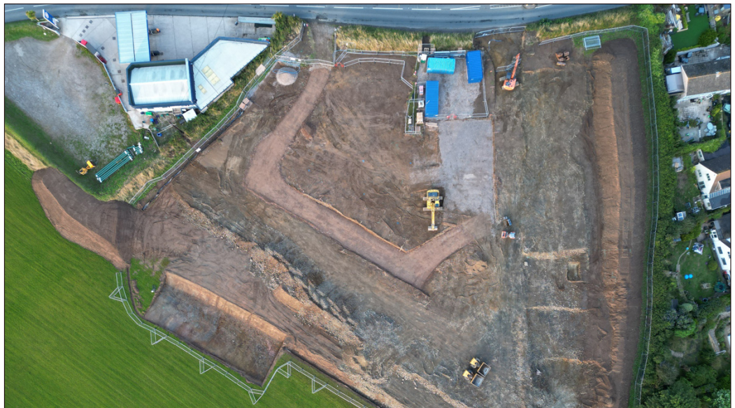
Work on the Salcombe site began before pre-commencement conditions were complied with
