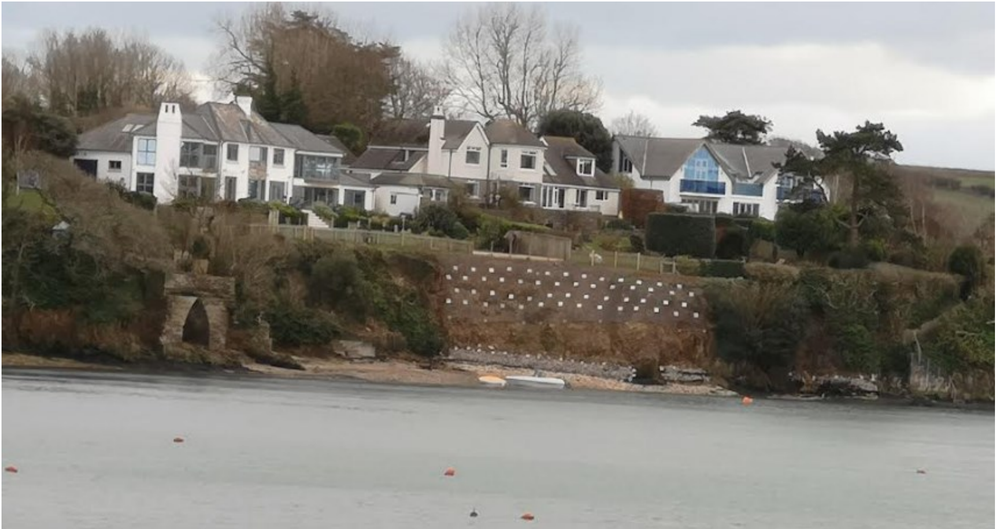
Image 2021 - estuary bank collapses in early 2019. Netting secured with rock bolts with stone gabion baskets along the base.
